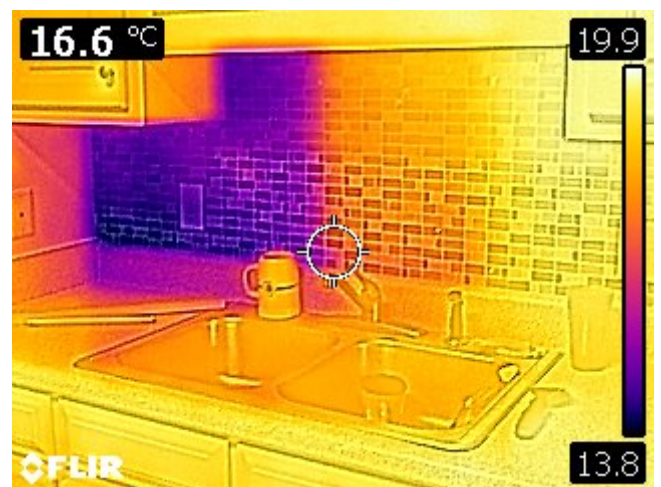
Figure 3: An exterior door with poor weather stripping (top), and an improperly insulated kitchen backsplash (bottom).
