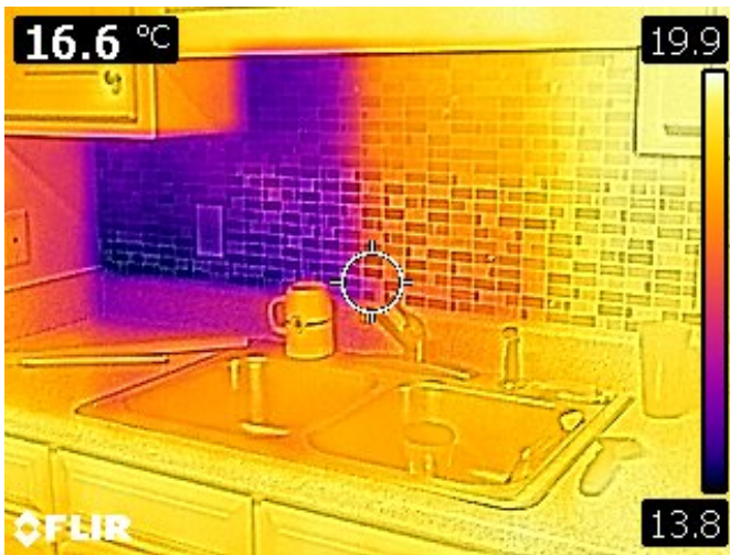
Fig. 4: A typical IR image taken with a FLIR C2, with the MSX image fusion option enabled. The image shows a kitchen backsplash on a wall with a poorly insulated fireplace behind it. The dark area in the upper left indicates a colder region, due to insufficient or missing insulation.
