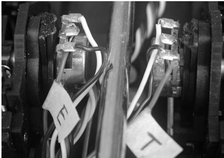
Figure 8. Potentiometer Detail of the Transmitter
